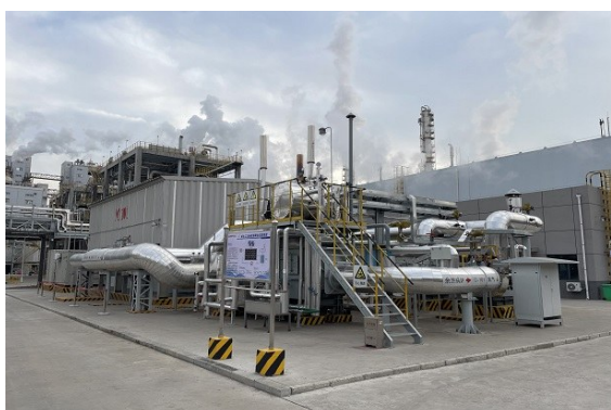
图 11 国家能源集团低碳院超高温炭基固体储热装置 [102] Fig. 11 Ultra-high temperature carbon-based solid thermal energy storage device from CLDR of CHN Energy [102]
